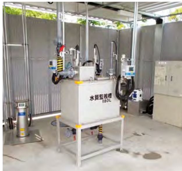
Water quality monitoring equipment
